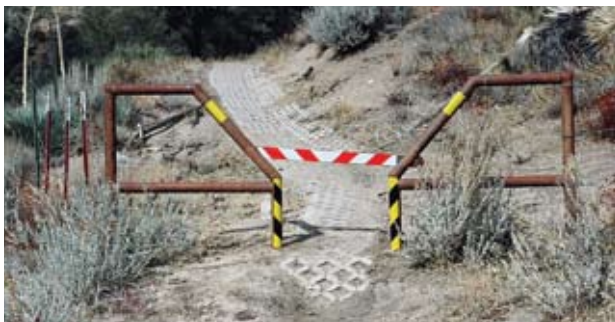
Figure B4. Use retroreflective red and white sheeting to highlight closure bar across trail.
