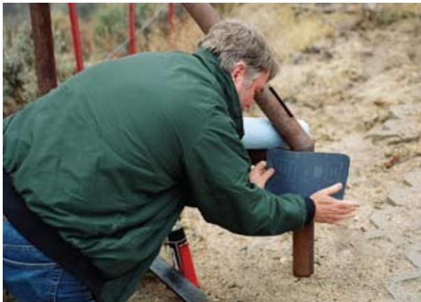
Figure B7. Sand the metal surface to remove rust and prepare a clean and smooth surface.
