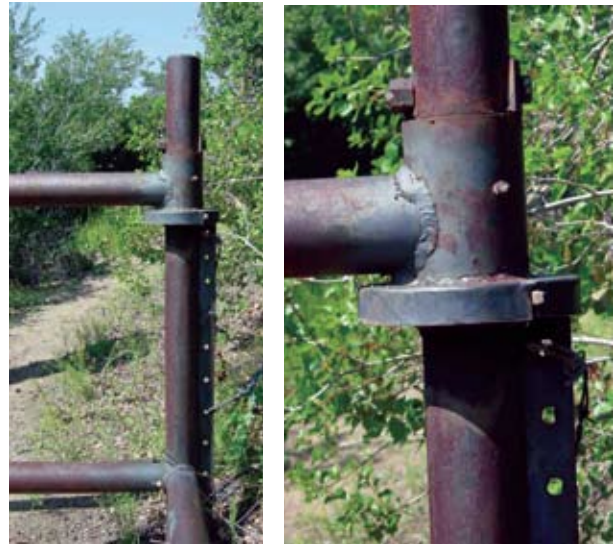
Figures 24 and 25. A barbed wire fence is strung through the holes on the flange on the side of the post. This prevents people from skirting the gate.
